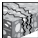
Concrete (cracked) a)
